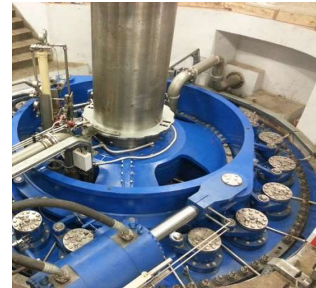
turbine HPP ZAKUČAC, Croatia
