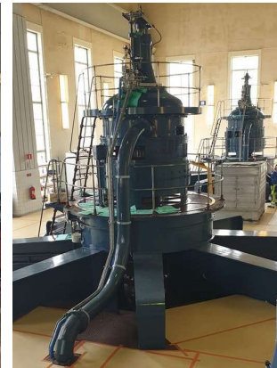
machine room HPP PUNTARIKOSKI, Finland
