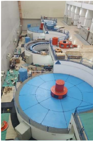
turbine HPP MOSTAR, Bosnia and Herzegovina
