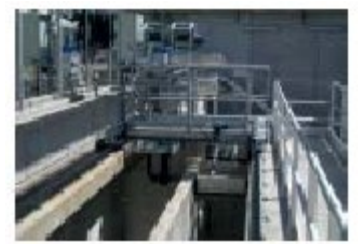
Sand Remover Bridges
